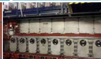
"Main LNG/Dual fuel engine"
