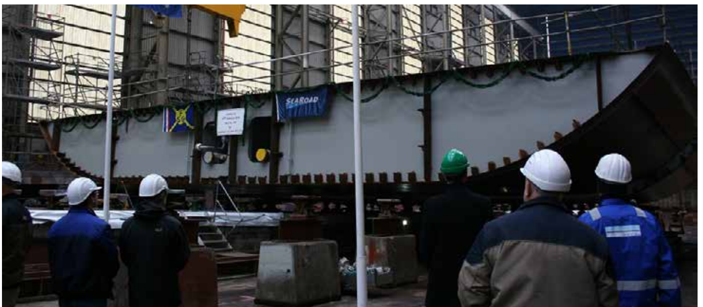
One of the three modules making up the keel in place at FSG's Flensburg Shipyard
