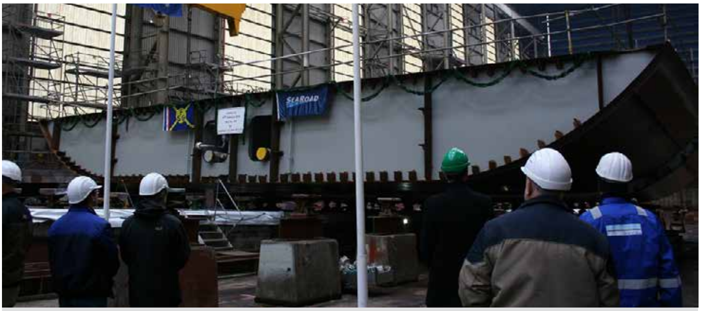
One of the three modules making up the keel in place at FSG's Flensburg Shipyard
